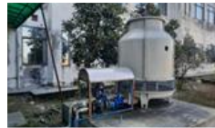
Cooling tower for indoor and outdoor cooler
