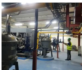
Energy Audit of Compressors
