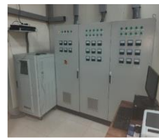
CONTROL PANEL FOR AC TESTING LAB
